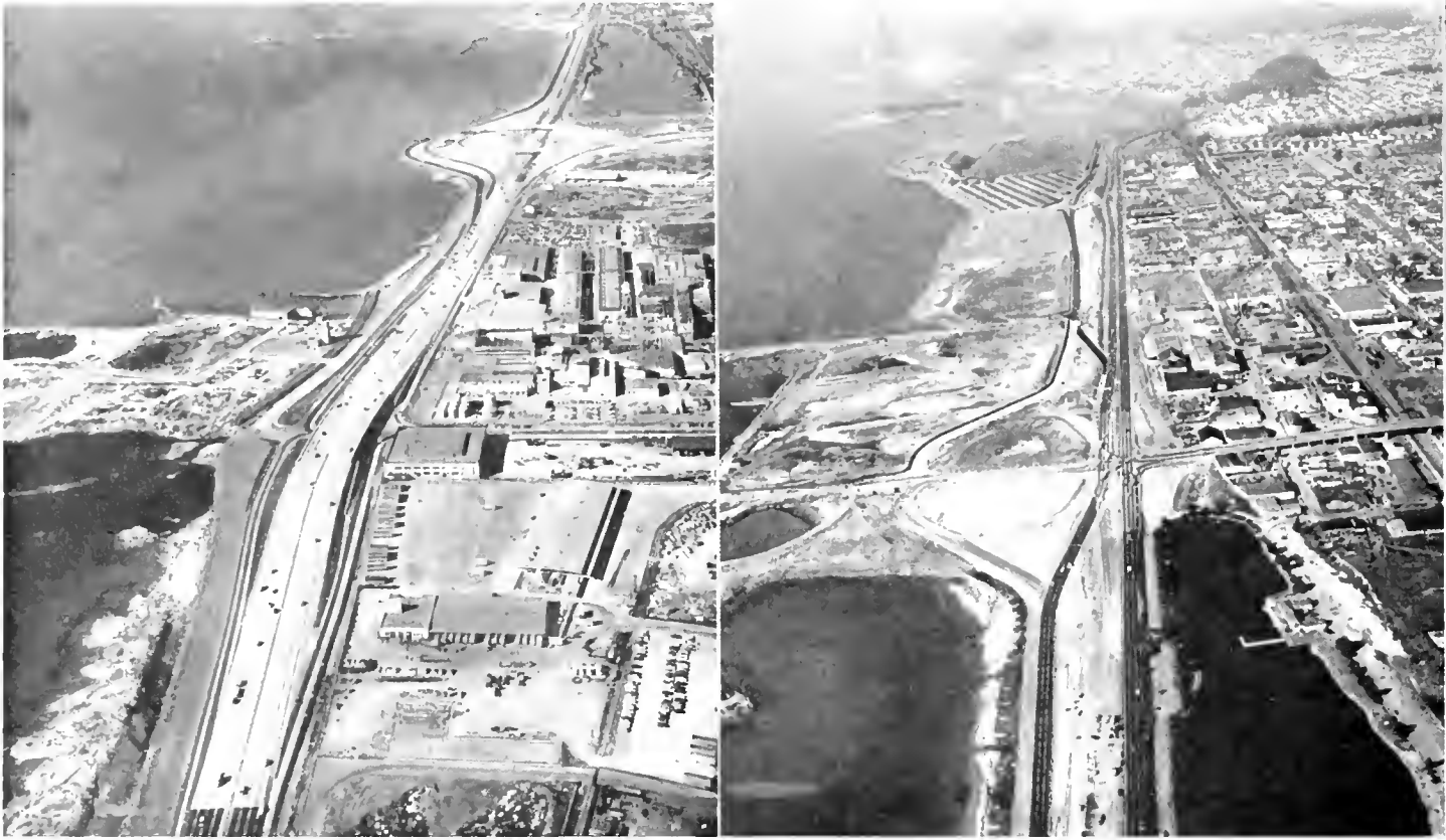
LEFT—View of the first completed unit of the Eastshore Freeway to the north of the distribution structure; Powell Street interchange in center; Ashby Avenue interchange beyond. RIGHT—View of construction operations for north section of Eastshore Freeway looking north from site of the University Avenue interchange toward the El Cerrito Overhead.
